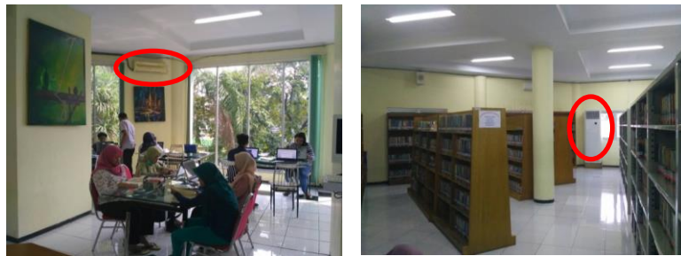
AC Split wall
